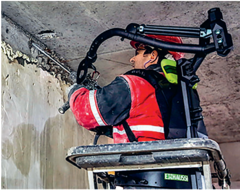
Testing an exoskeleton designed to reduce the risks associated with carrying tools and to facilitate movements, during work to renovate a listed mansion in Rue de Courcelles, Paris.
