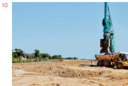
10 Foundations for the future Ariane 6 launch pad at the Guiana Space Centre in Kourou.
